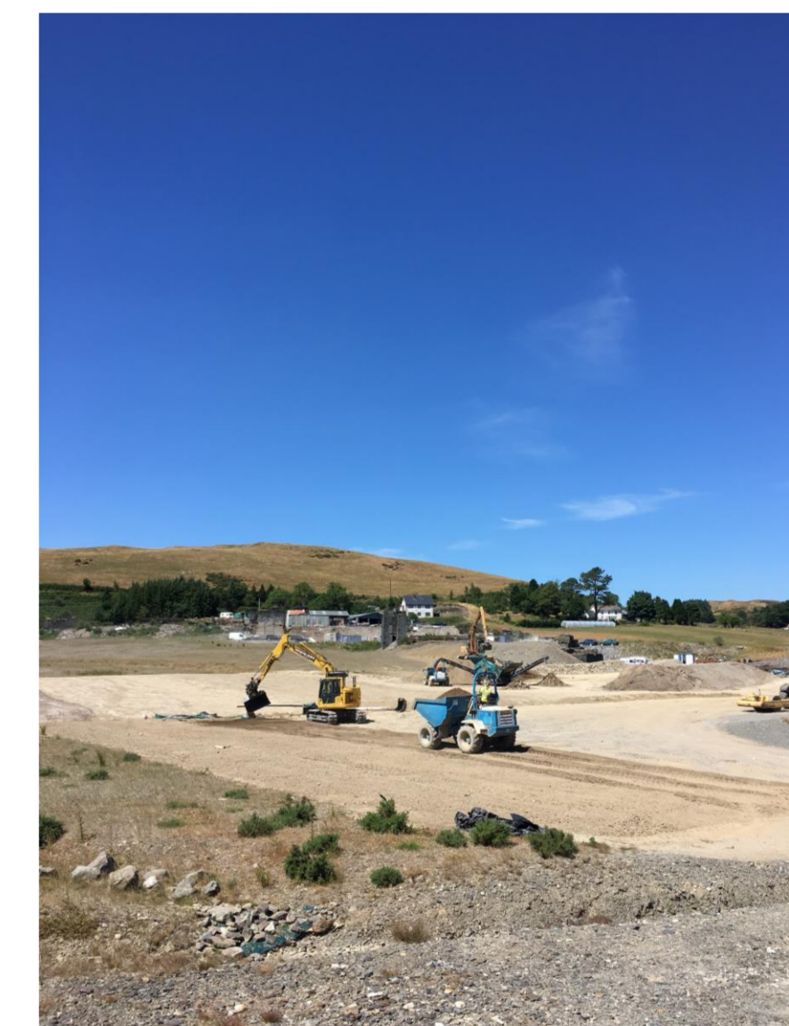
Figure 5. Covering the geosynthetic clay liner with a minimum 100mm blinding layer of material to inhibit the potential for puncture or damage by angular material.
