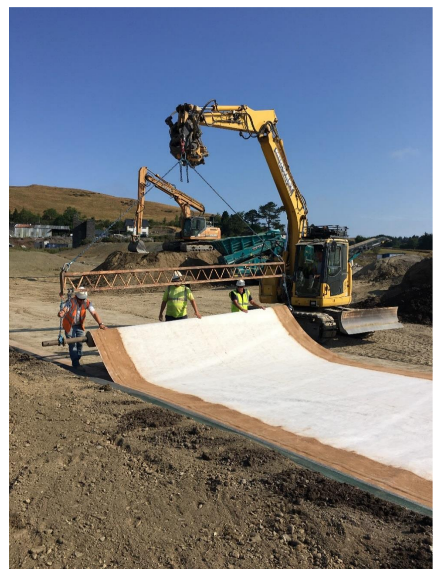
Figure 3. Deployment of the geosynthetic clay liner using a suspended I-beam and excavator.
